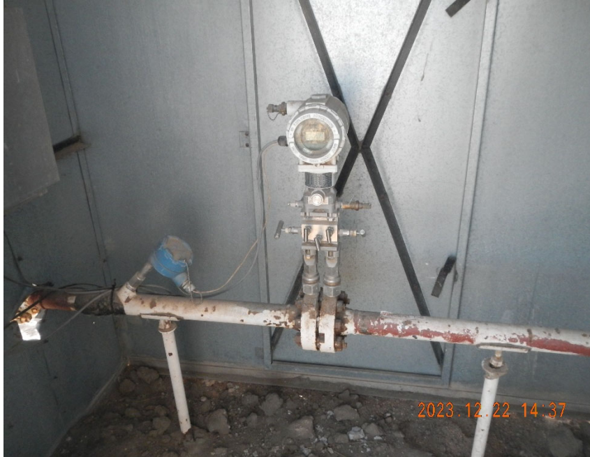
5. Digital gas meter inside meter shed.
