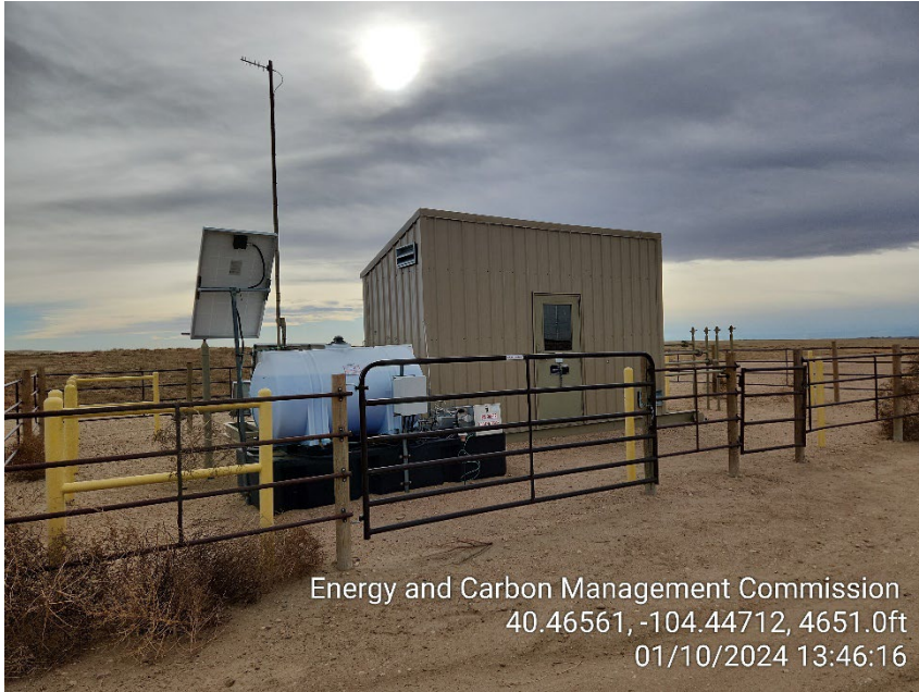
Photo 5 – Gas Lift Injection Meter House
