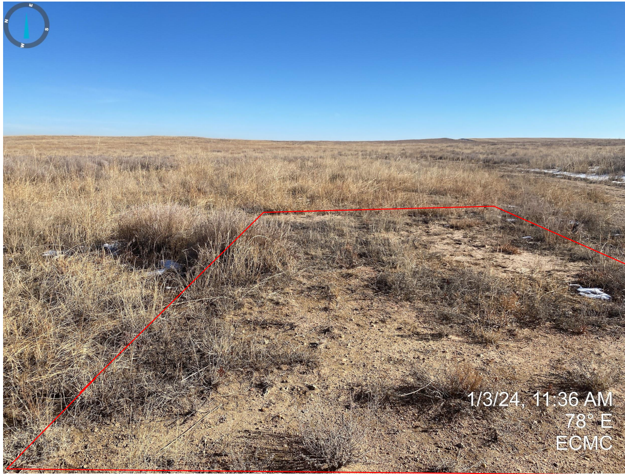
Photo 4. Taken from the western portion of the former well. Non-uniform vegetative cover at the former well location. Additional reclamation activities are required.
