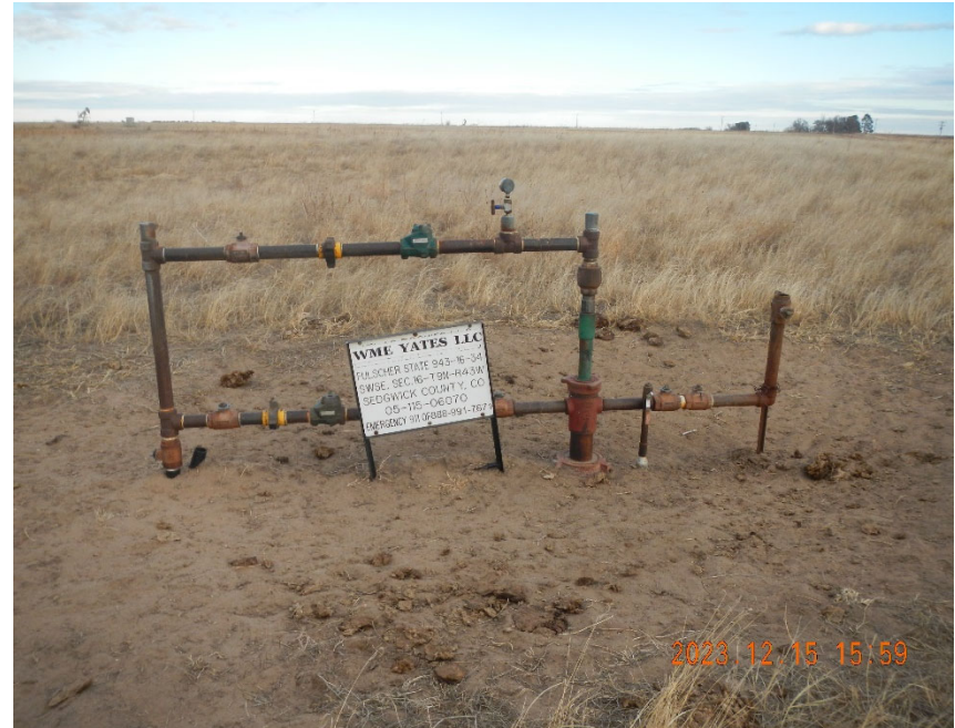
2. View of wellhead.
