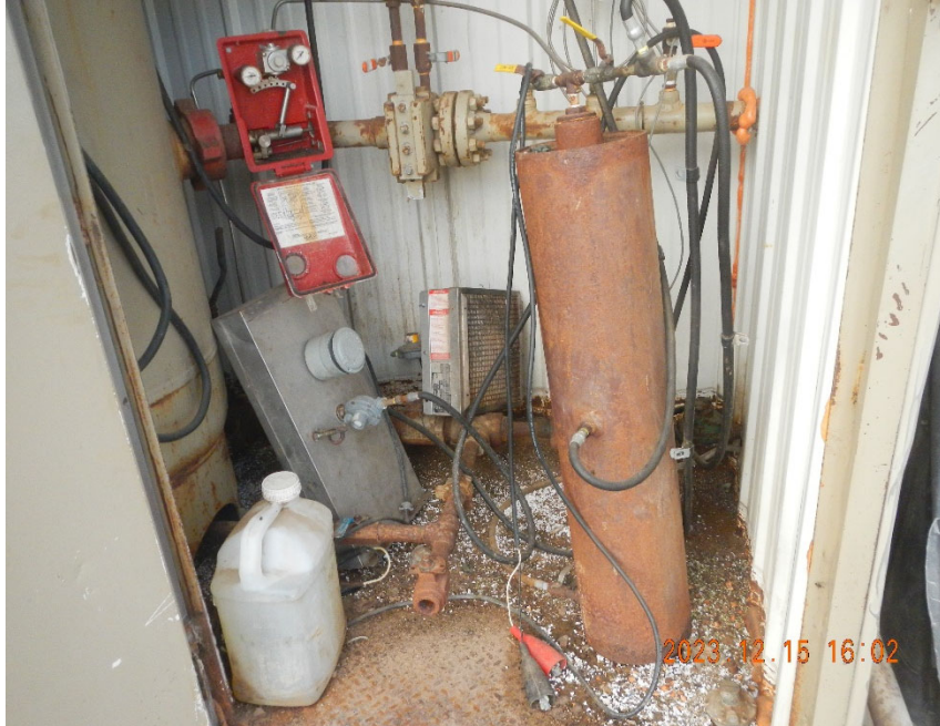
5. Vertical separator, meter, and heater inside meter shed.
