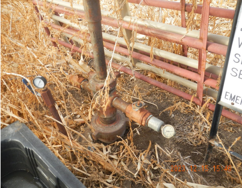
3. Additional view of wellhead.
