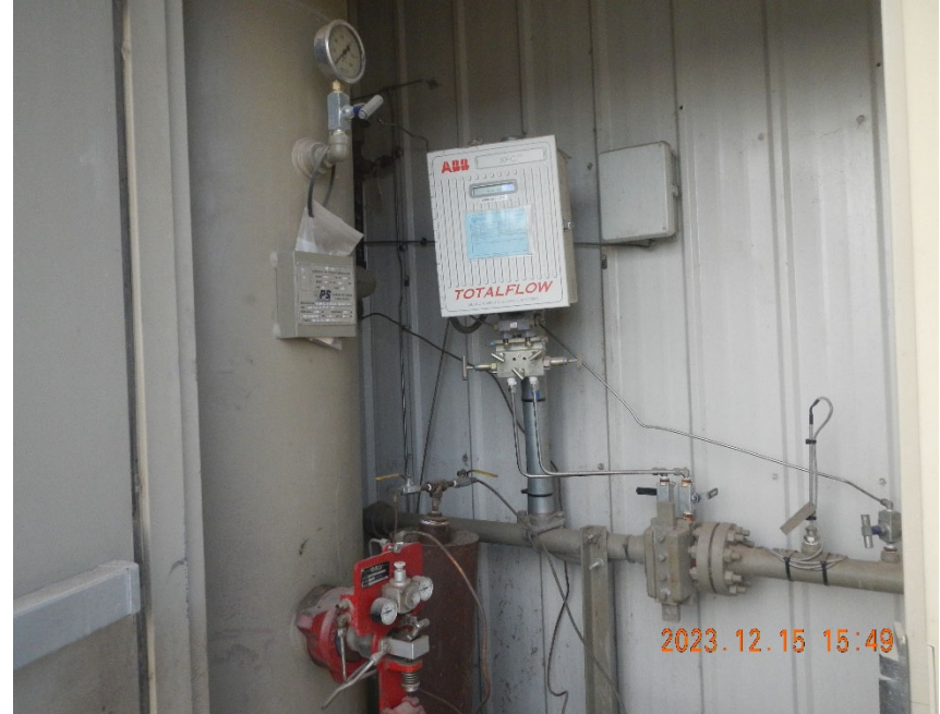
6. Vertical separator and gas meter inside meter shed.
