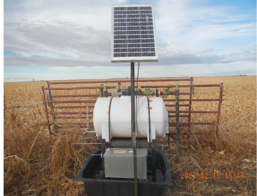
4. Chemical tank and pump at wellhead.
