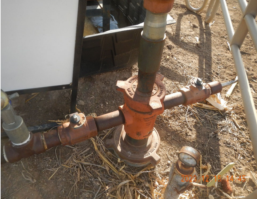
3. Additional view of wellhead.
