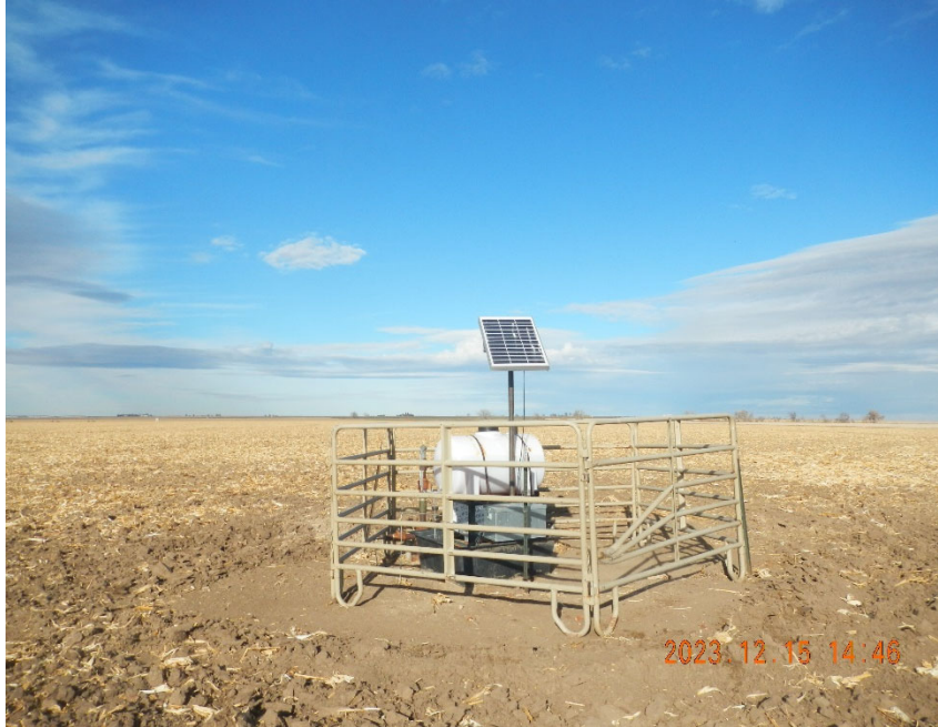
5. Well site overview.
