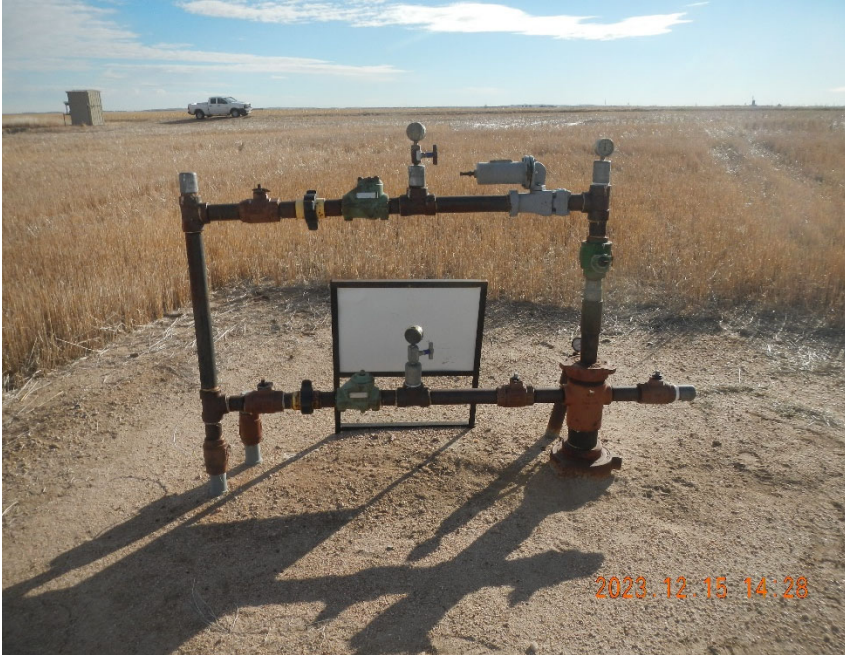
3. Additional view of wellhead.
