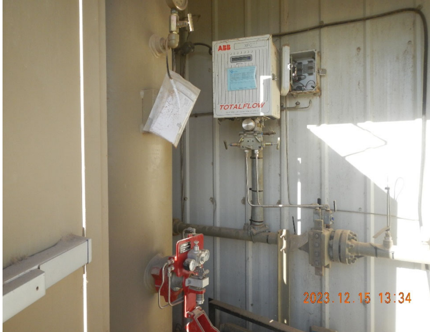
5. Vertical separator and gas meter inside meter shed.
