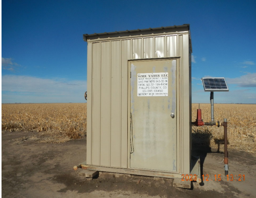
3. Meter shed. Door is jammed closed and unable to access.
