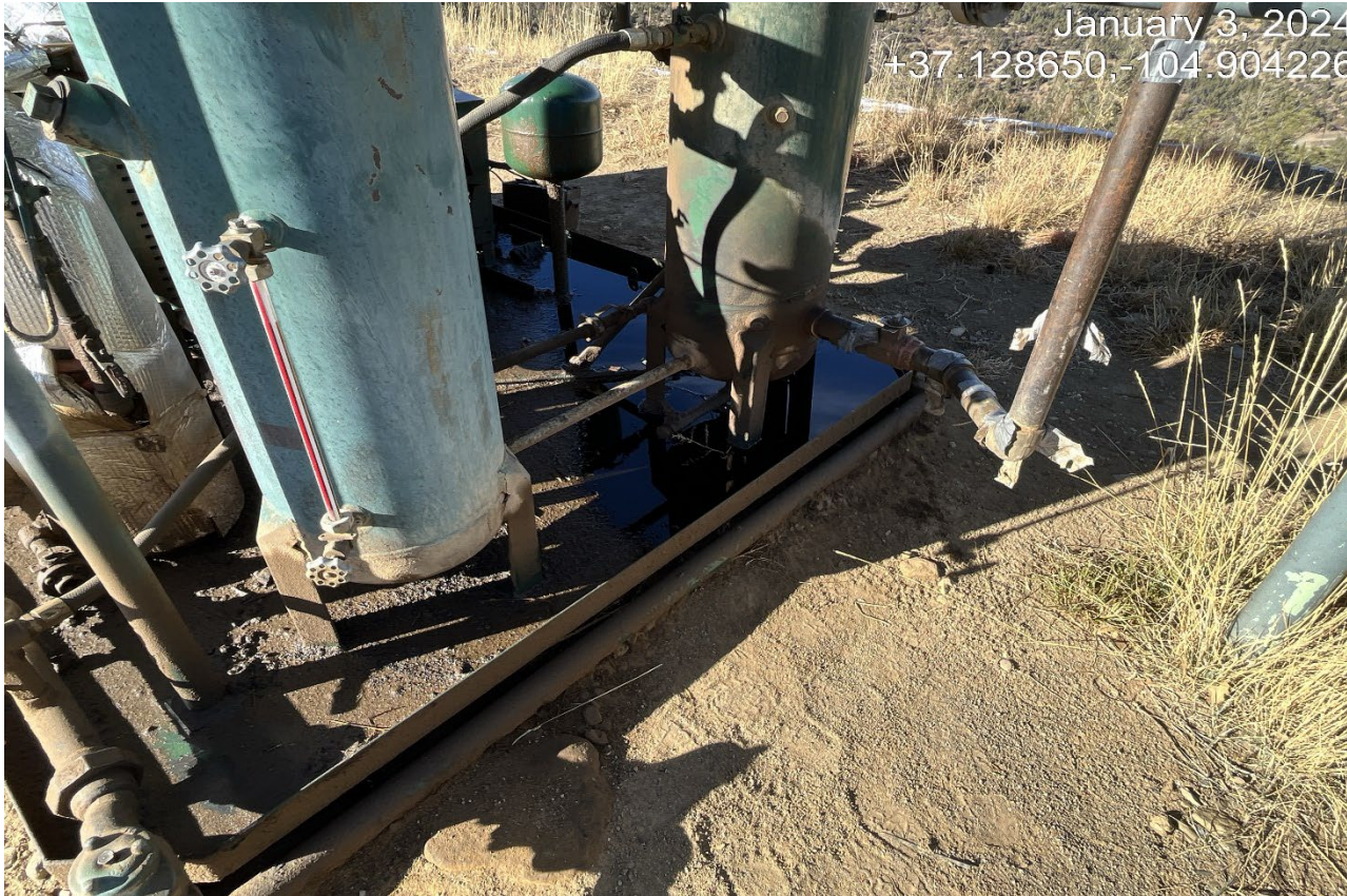
Photo 2. There is oil in the engine skid that needs to be cleaned up.
