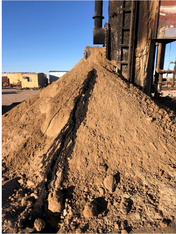
1. Oil leaking from Treater before vac truck
