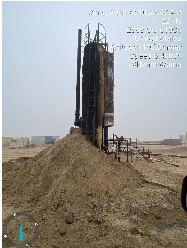
3. Scorched insulation on west side
