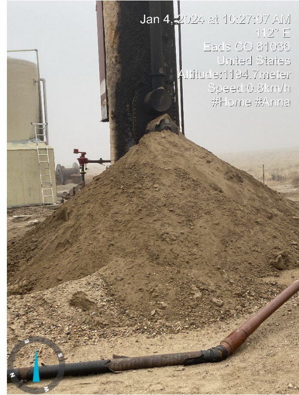
2. Oil cleaned up, filled a 5 gallon bucket
