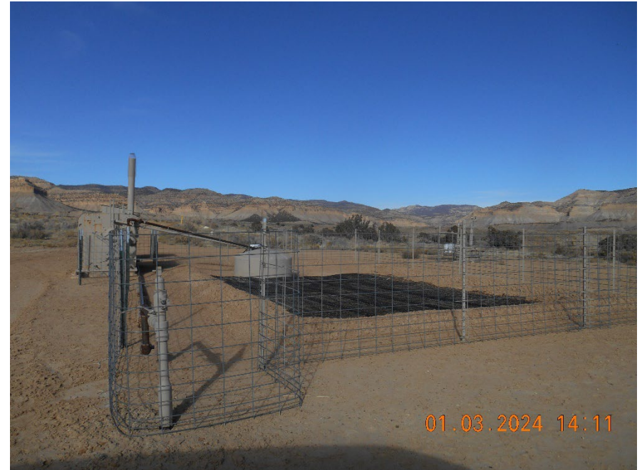
Tank Battery and Blowdown Pit
