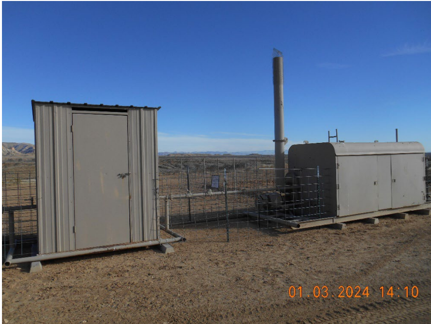
Separator and Meter Housing
