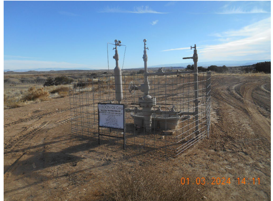
Wellhead with fence and sign
