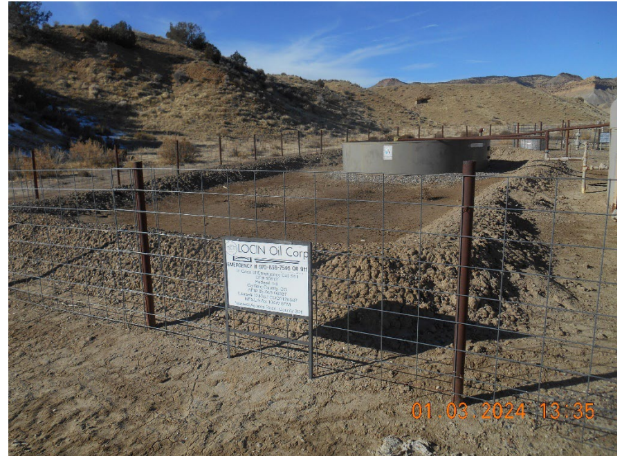
Tank Battery with fence and berms
