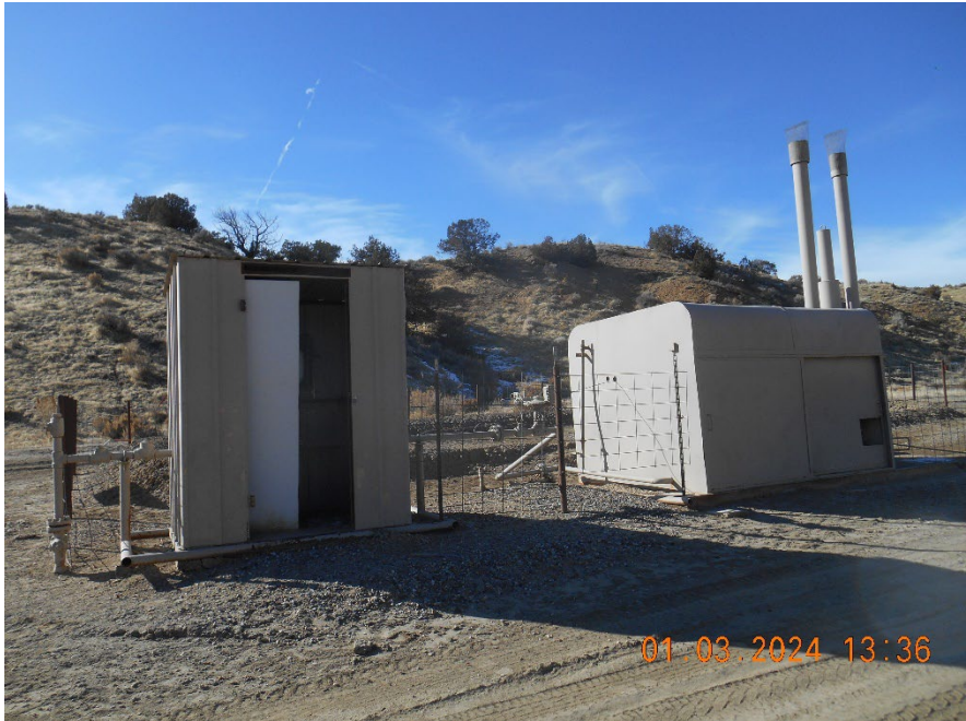
Separator and Meter Housing
