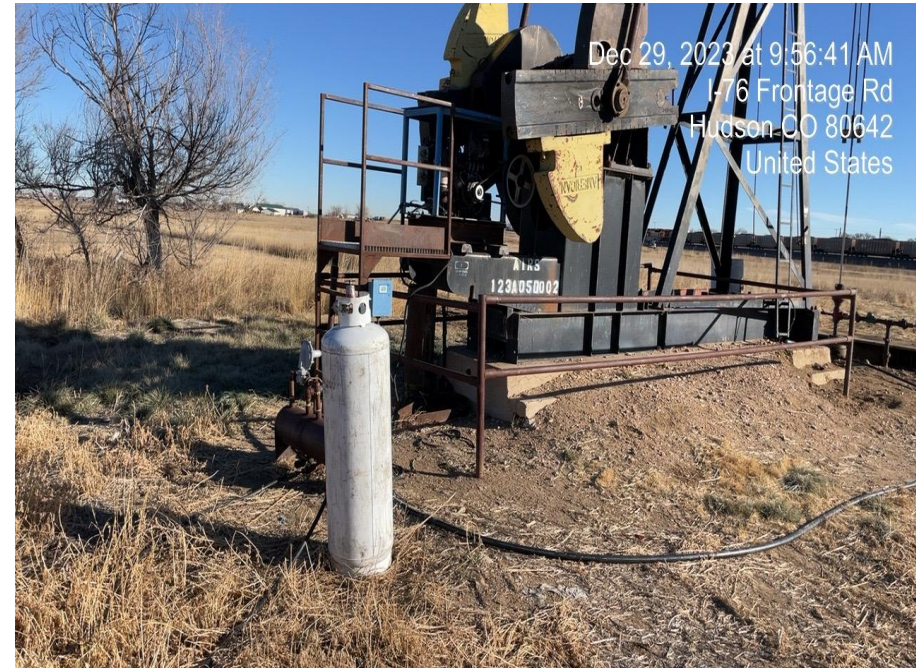
Photo 6. Photo of propane tank attached to pumping pumpjack. Photo tank facing northeast.
