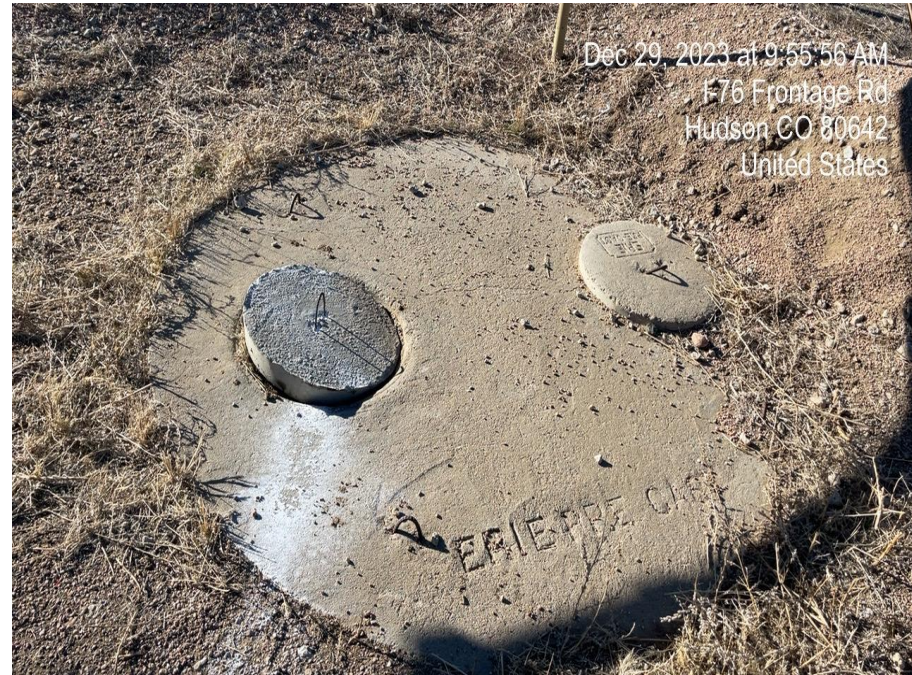
Photo 4. Photo taken of equipment buried tank in tank battery. Photo taken facing west.
