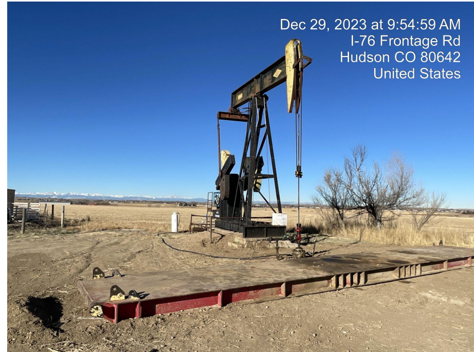
Photo 2. Photo taken of operating Wellhead. Photo taken facing west.
