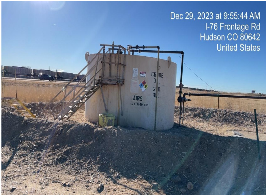
Photo 3. Photo taken of tank battery. Photo taken facing west.
