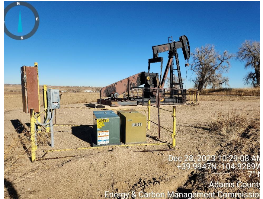
Photo 4 pumping unit and equipment
