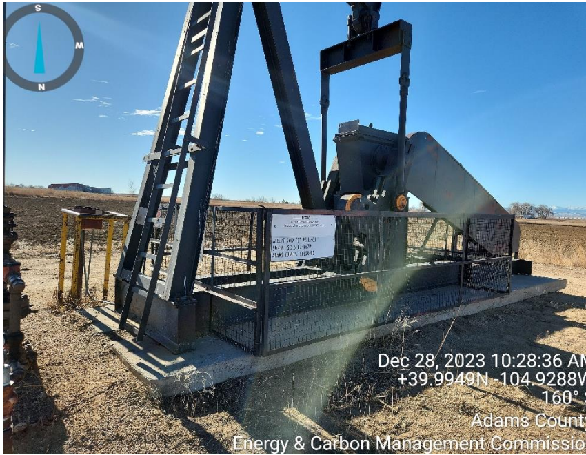
Photo 3 pumping unit with sign
