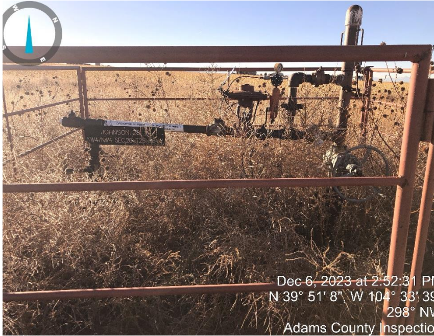
Photo #5 well head
