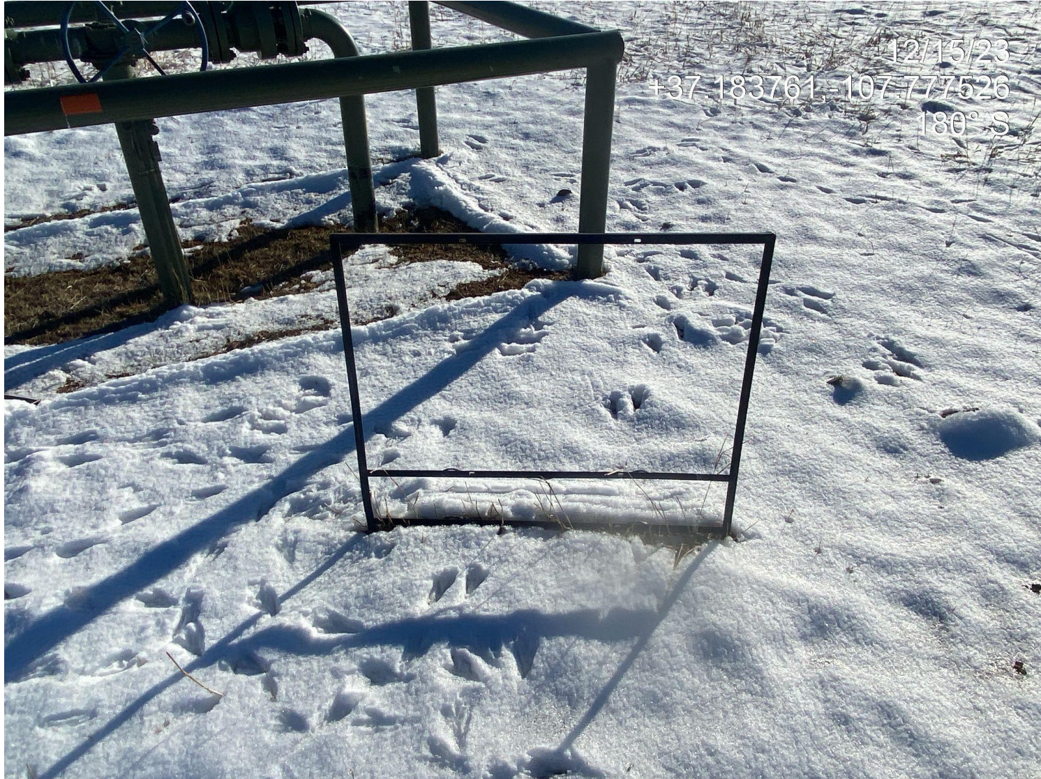
Photo 3. View of sign missing from location.
