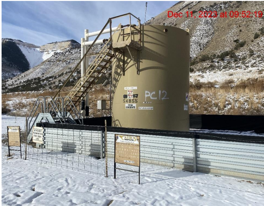
Tank Battery – Photo #08051
