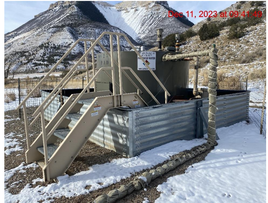
Tank Battery – Photo #08038
