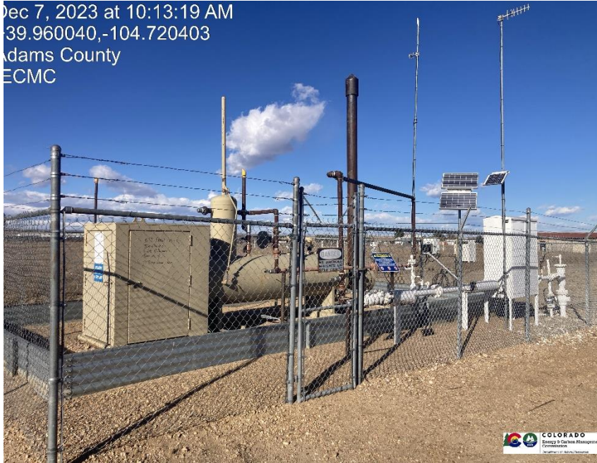
Pic 3 Separator, GMR
