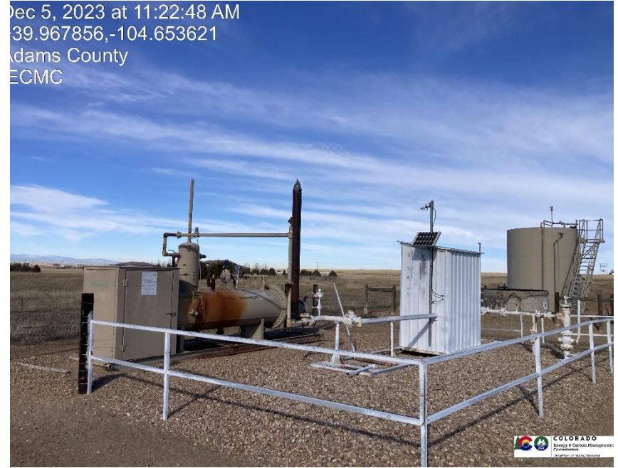
Pic 2 Separator, GMR
