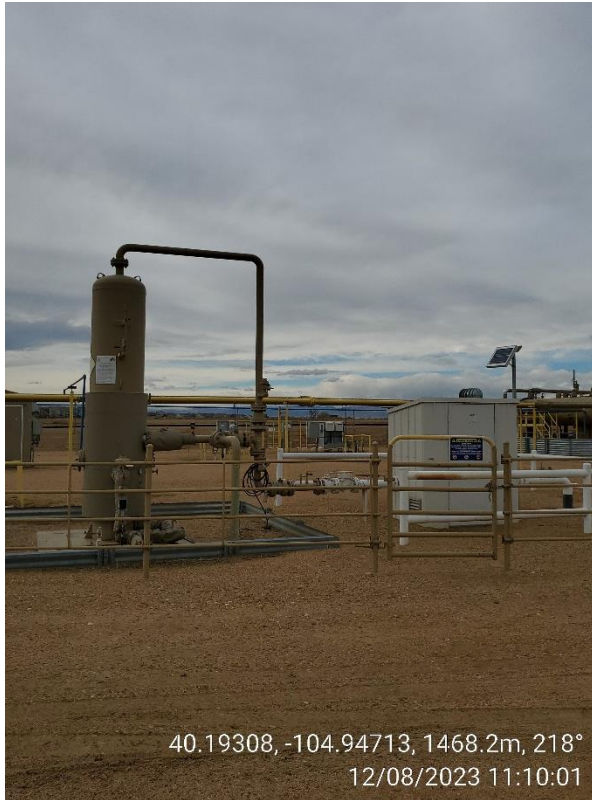
Photo 7 Vertical Separator and GMR
