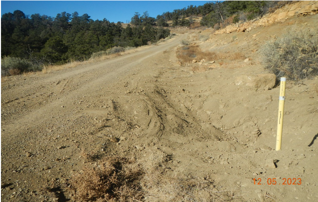
Photo 1. Facing northwest along the main road. The culvert has been cleaned out. This area should also be seeded for stabilization.
