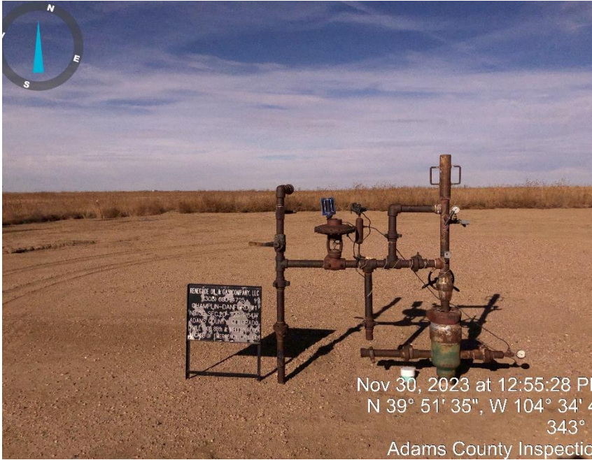
Photo #3 Well head.
