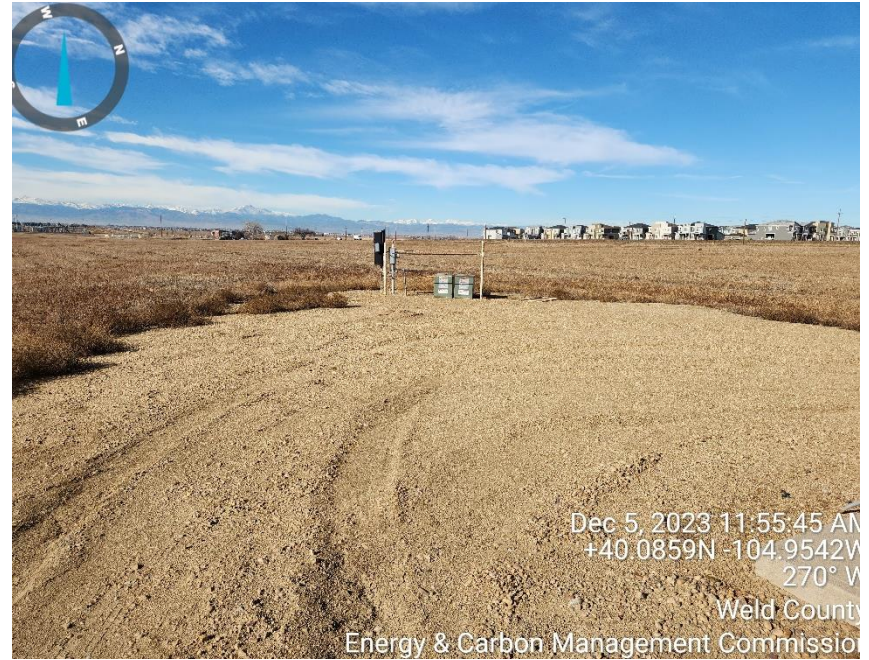
Photo 2 electrical disconnect panel
