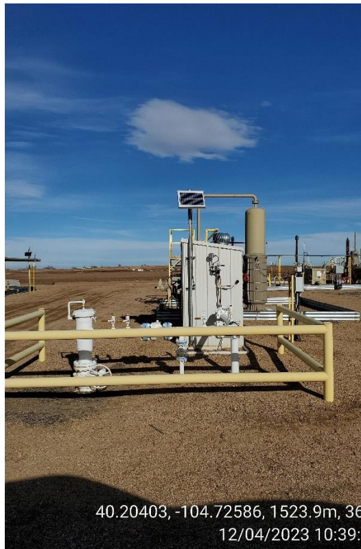
Photo 2 GMR and Pig Station
