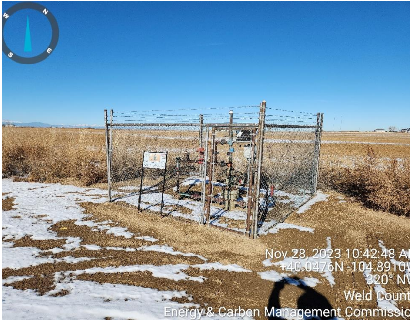
Photo 1 well head and equipment
