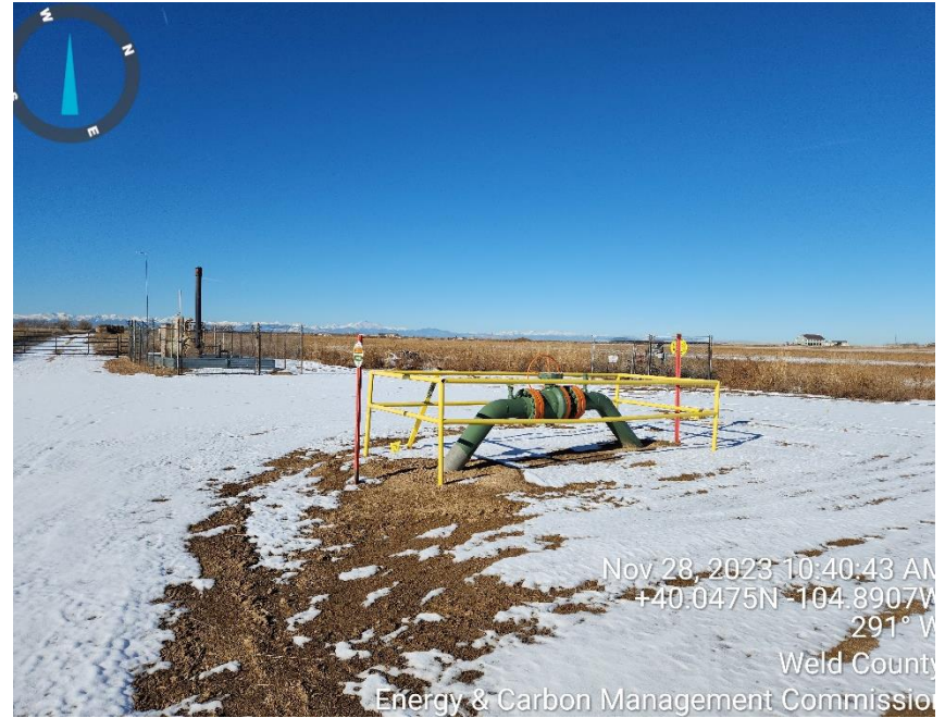
Photo 4 pipeline crossing valve riser
