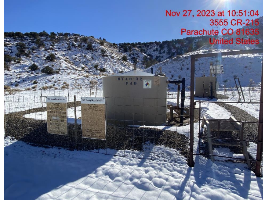
Tank Battery – Photo #07696
