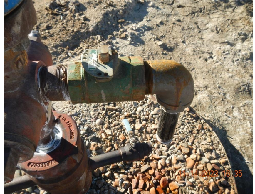
Drips from this valve could be seen once every 10-15 seconds.
