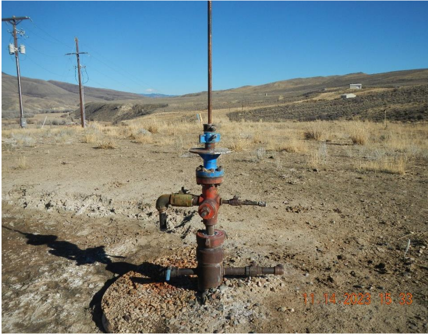
2 inch valve on the upper left of the well head dripped once every 10-15 seconds.
