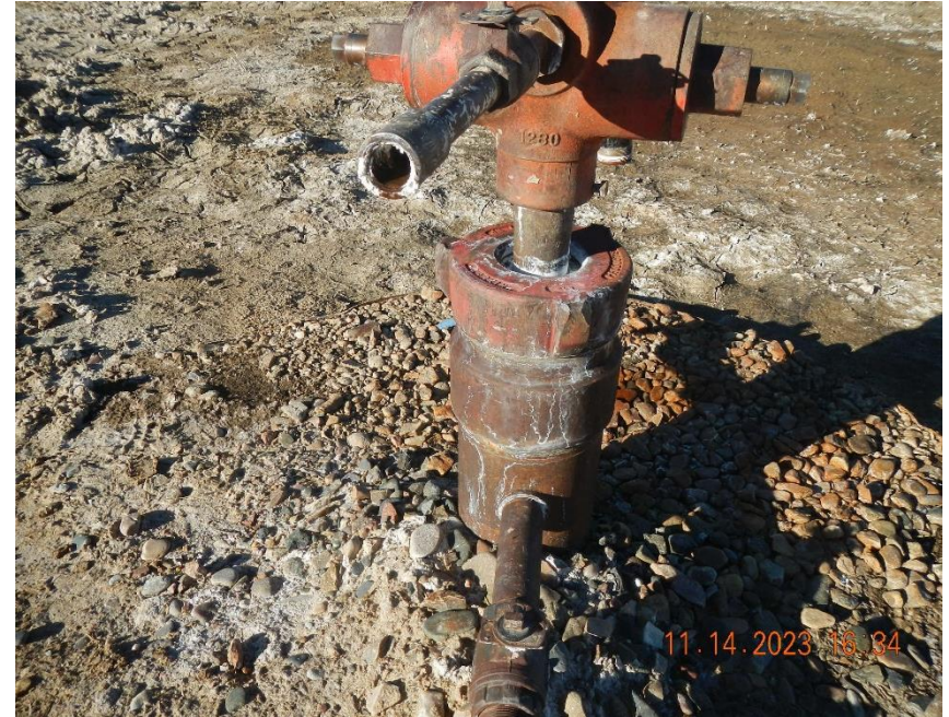
One inch valve is wet and stained.
