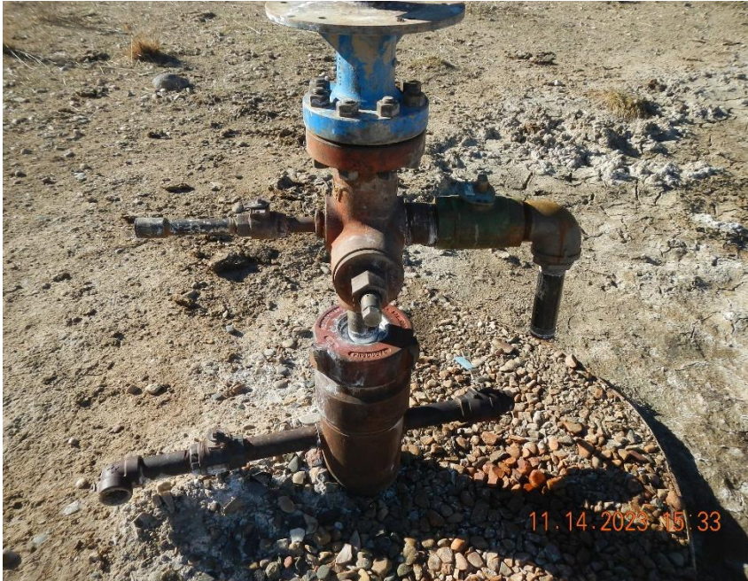
Close up of BM Federal #13-12 well head. All valves appeared to be in the closed position during this inspection.
