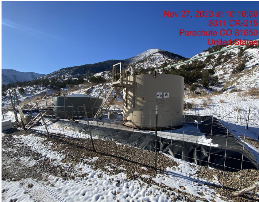
Tank Battery – Photo #07663
