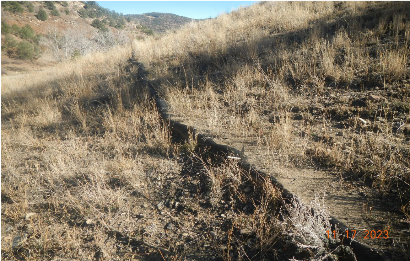
Photo 3. Facing east along the upper slope. The erosion wattles will need to be removed for final reclamation.
