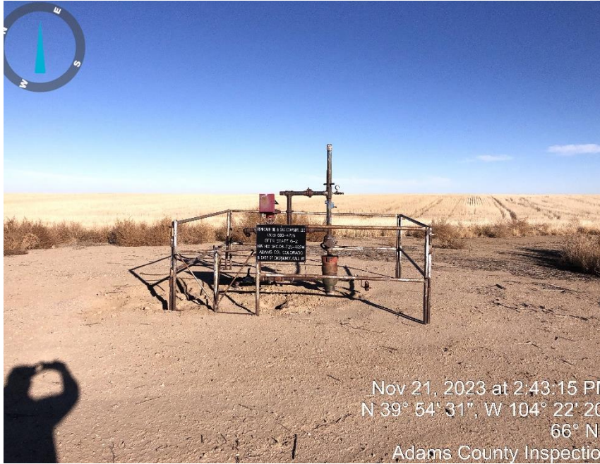
Photo #1 Well head.
