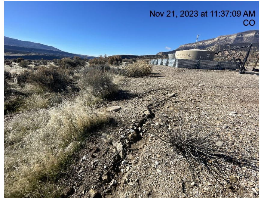
Photo # 7232 Erosion & transport of sediment off location
