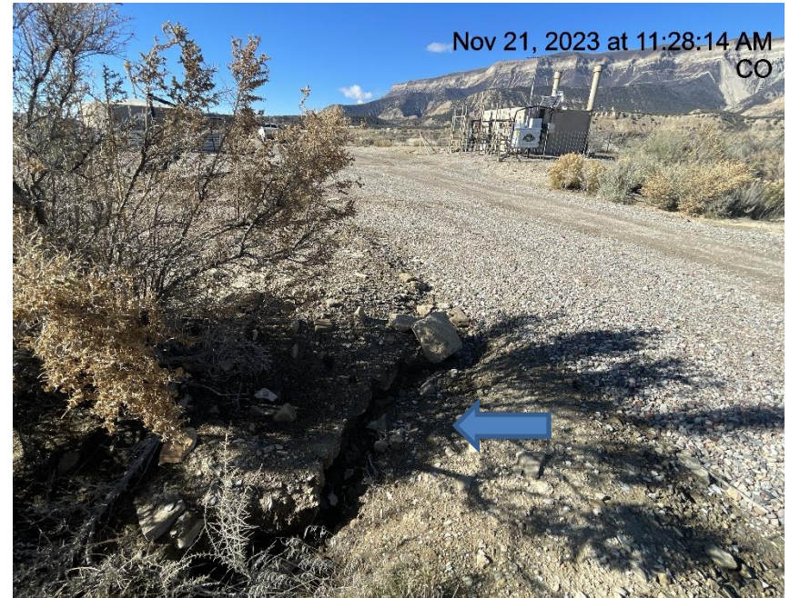
Photo # 7226 Erosion & transport of sediment off location
