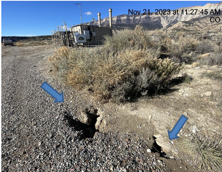
Photo # 7225 Tunnel erosion
