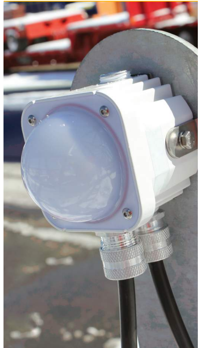
The Cube-Light on an STS crane
