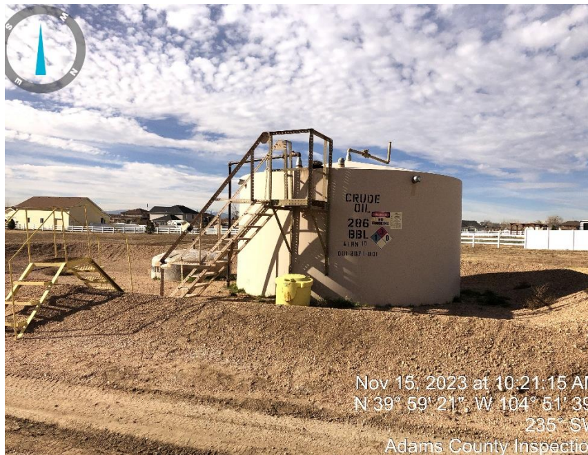
Photo #1 Crude tank.
