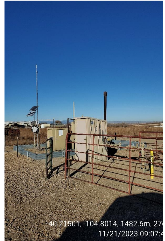
Photo 3 Separator, GMR and Pig Station
