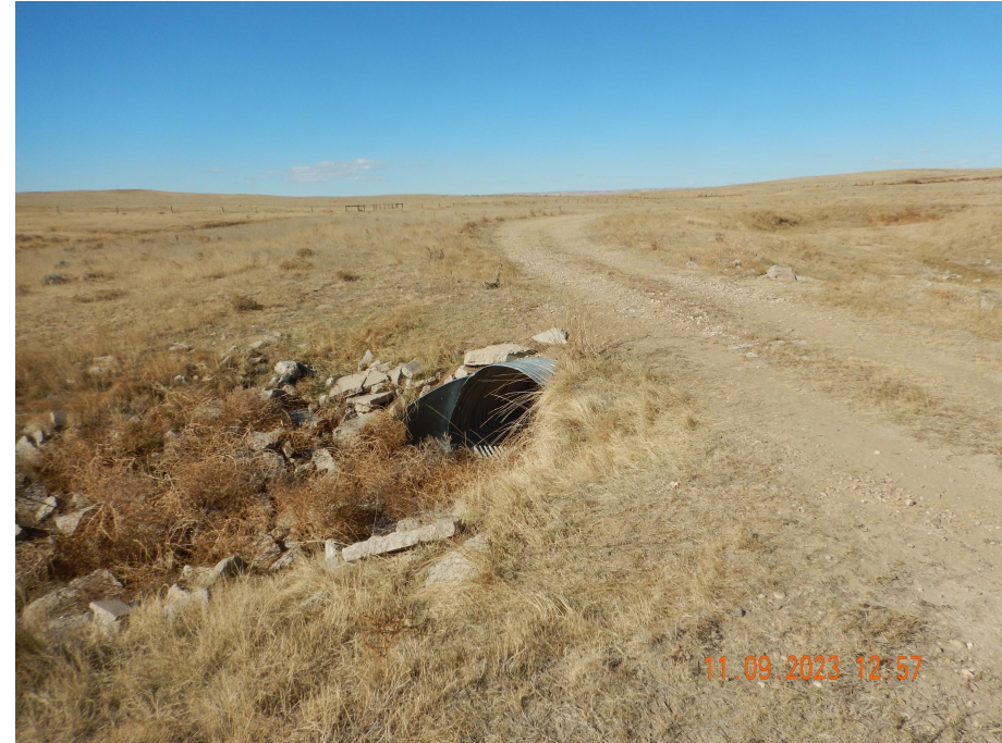
Photo 3. Photo taken from the drainage crossing, facing Northwest. Photo illustrates a culvert remains. Operator is coordinating with the Forest Service on plans to remove the culvert.
