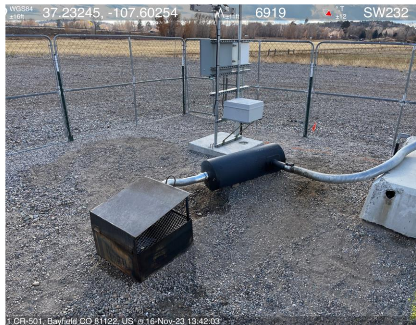
Photo #2. View of unresolved impacts from corrective action.
