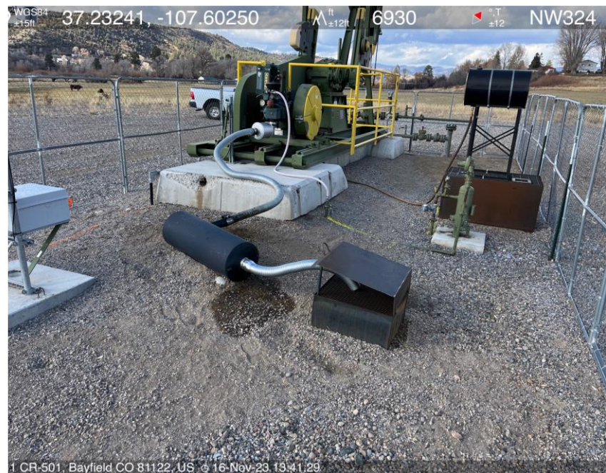
Photo #4. View of unresolved impacts from corrective action.
