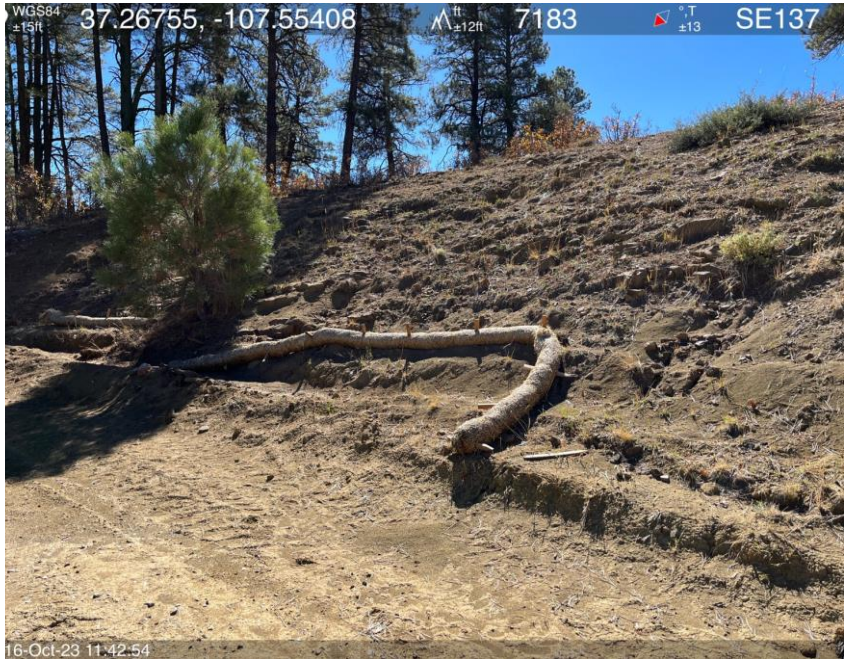
Photo #3. . View of corrective action identified in FIR Doc.#712700749.
