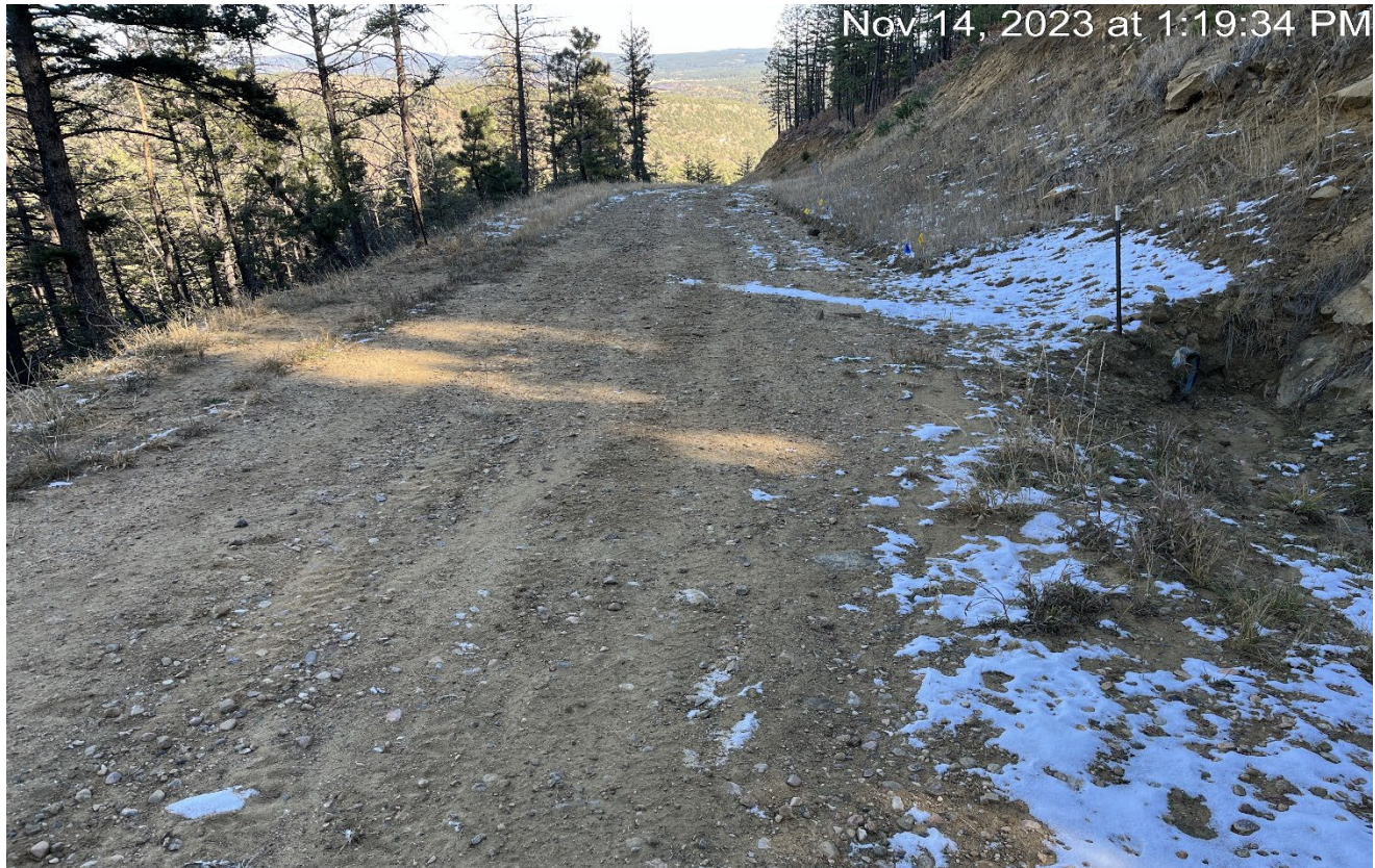
Photo 1. Facing east along the access road. Areas of erosion were repaired and culverts have been cleaned out..
