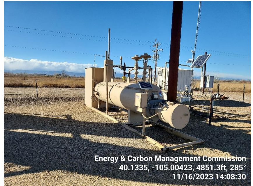
Photo 8 Horizontal Heated Separator.
