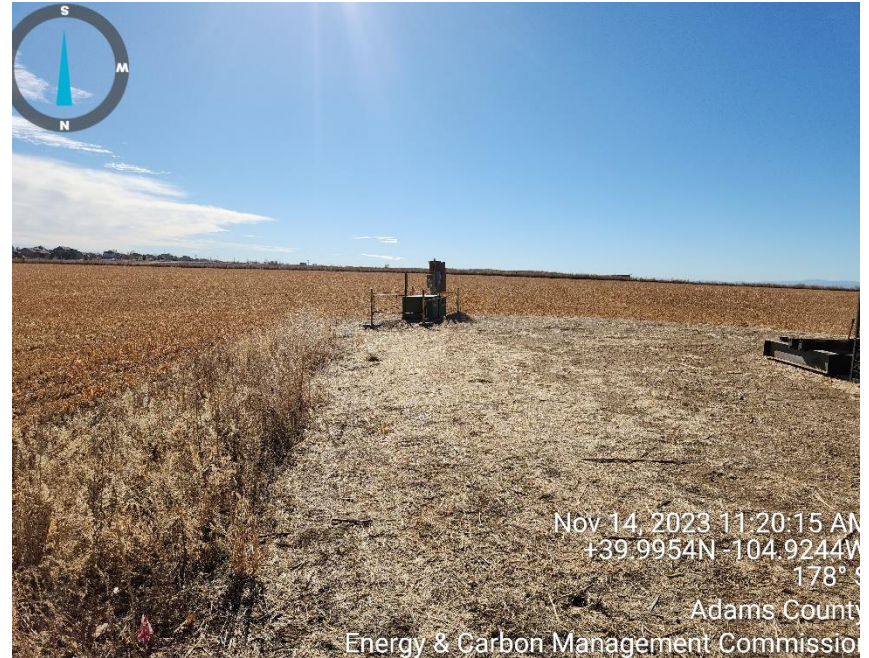
Photo 4 electrical disconnect panel
