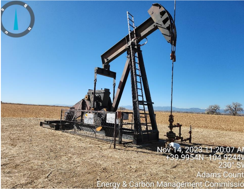
Photo 1 well head and equipment
