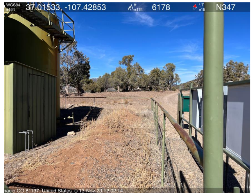
Photo #4. Corrective action not completed.
