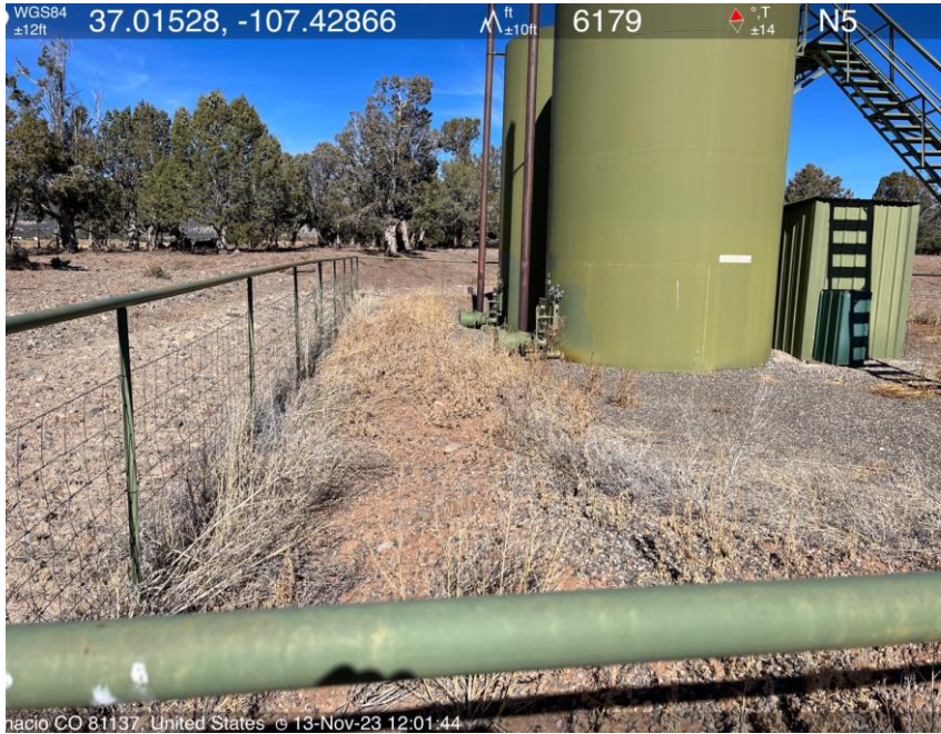
Photo #3. Corrective action not completed.
