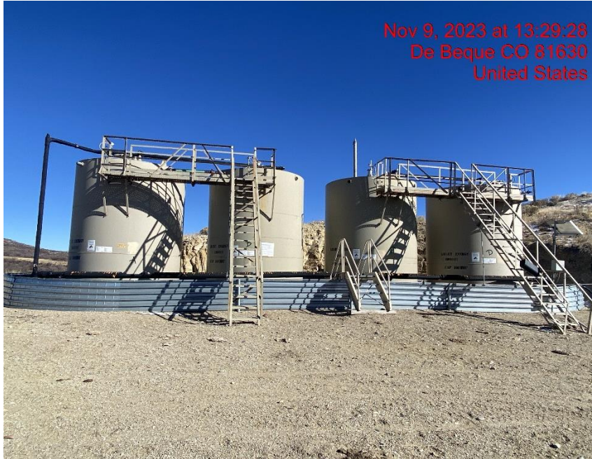
Tank Battery – Photo #07466
