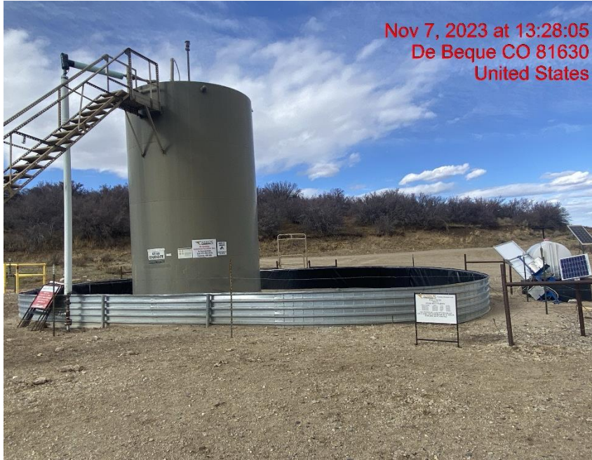
Tank Battery – Photo #07373
