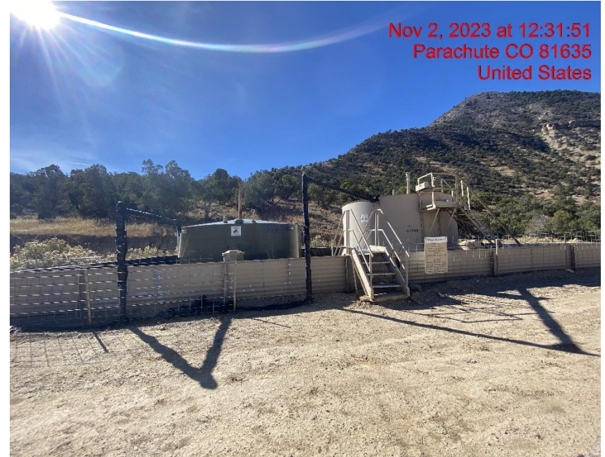
Tank Battery – Photo #07346
