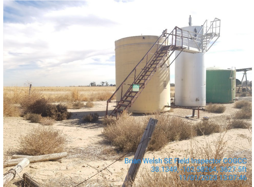
Northwest corner of tank battery
