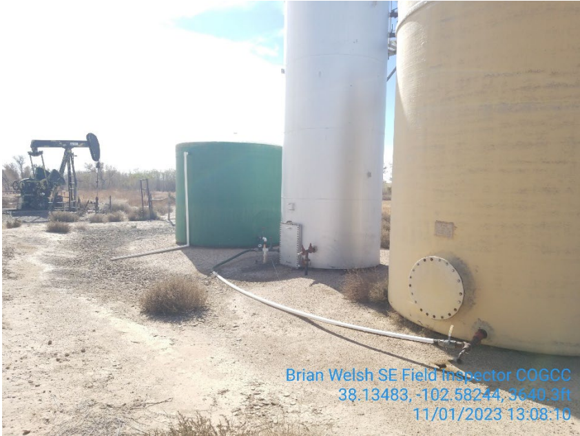
Northeast corner of tank battery
