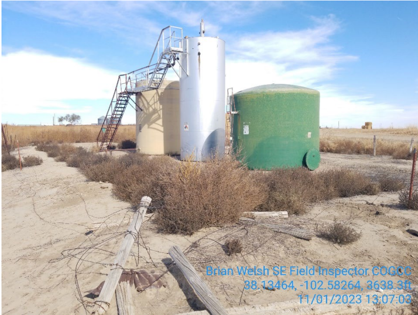
Southwest corner of tank battery
