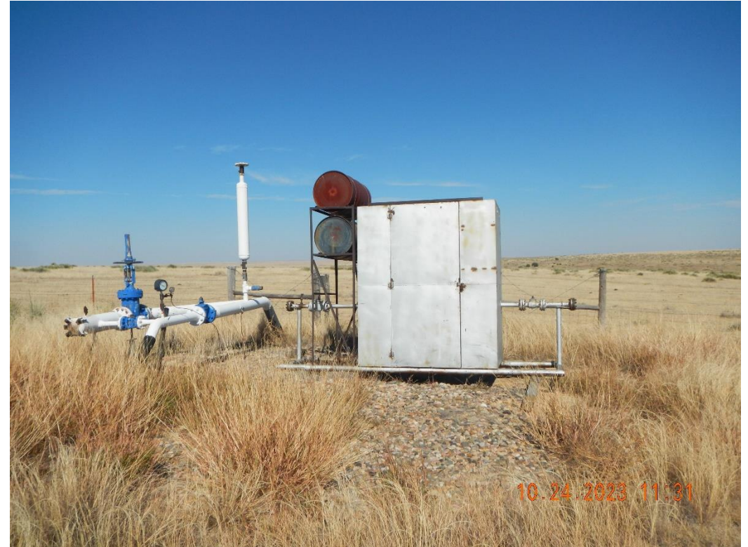
Pigging station on north side of location.
