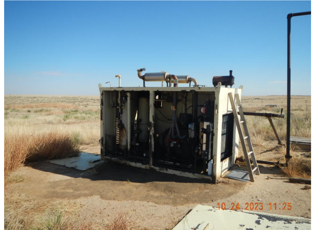
Stained ground from spill(s) at compressor.
