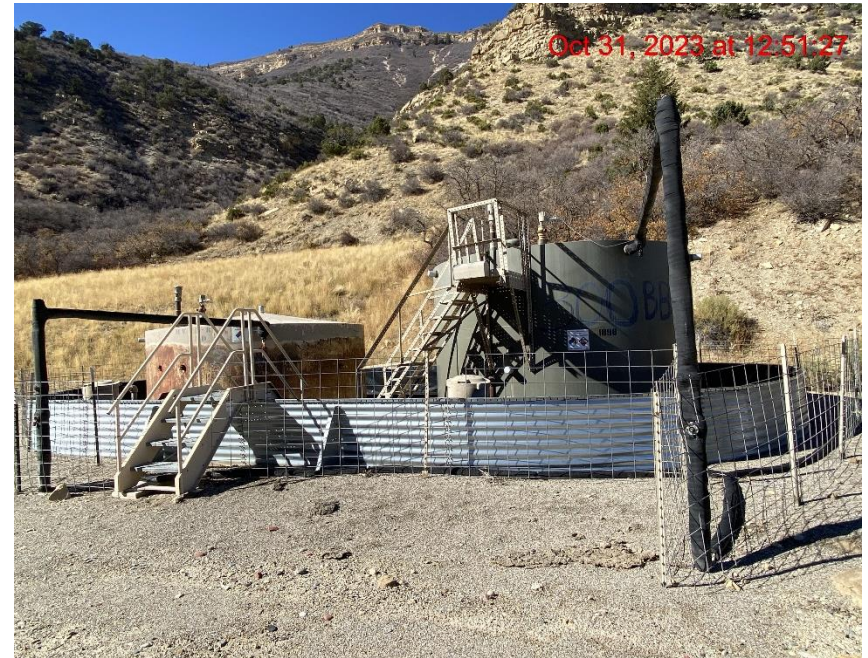
Tank Battery – Photo #07283
