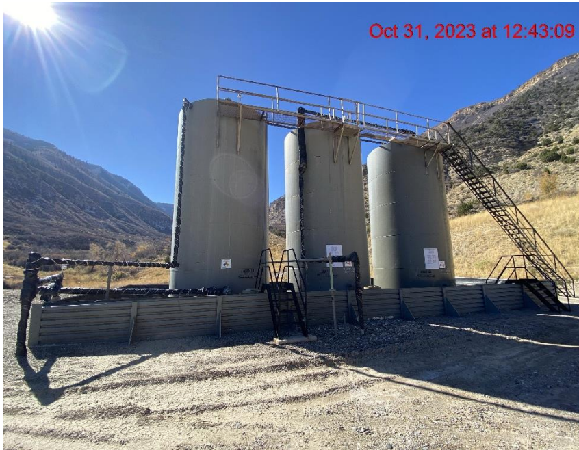
Tank Battery – Photo #07269
